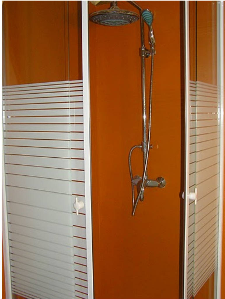
Bathroom with shower
